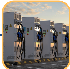
EV Public Charging
